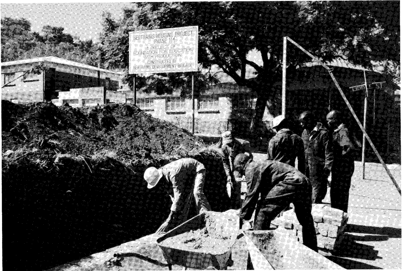
'On site, training began with clearing the site, marking the outline of the building and digging the foundation'
